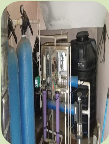
R.O. WATER PLANT
